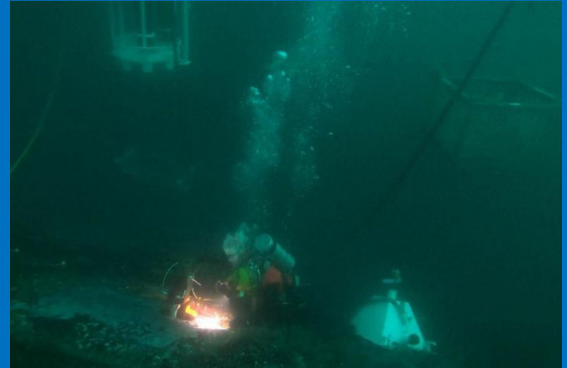
Divers securely drill into and access oil tanks of the wreck of the British-flagged tanker Coimbra on May 8, 2019.
